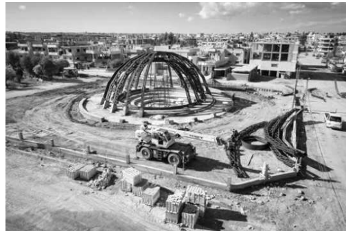
CONSTRUCTION OF THE NEW PUBLIC PARLIAMENT AND SURROUNDING PARK IN THE CITY OF DERİK, CEZİRE CANTON, IN THE AUTONOMOUS REGION OF ROJAVA IN EARLY DECEMBER, 2015. PHOTO: RUBEN HAMELINK/NEW WORLD SUMMIT.
